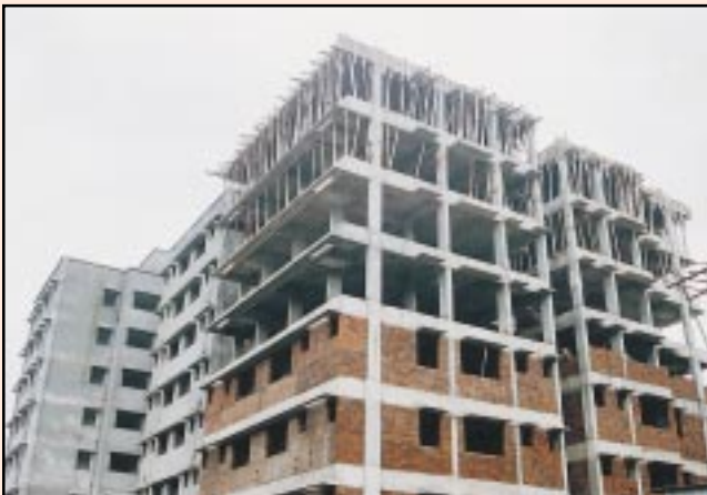
Building under Construction in the slum Rehabilitation Project by SPARC Samudaya Nirman Sahayak, Dharavi, Mumbai.
